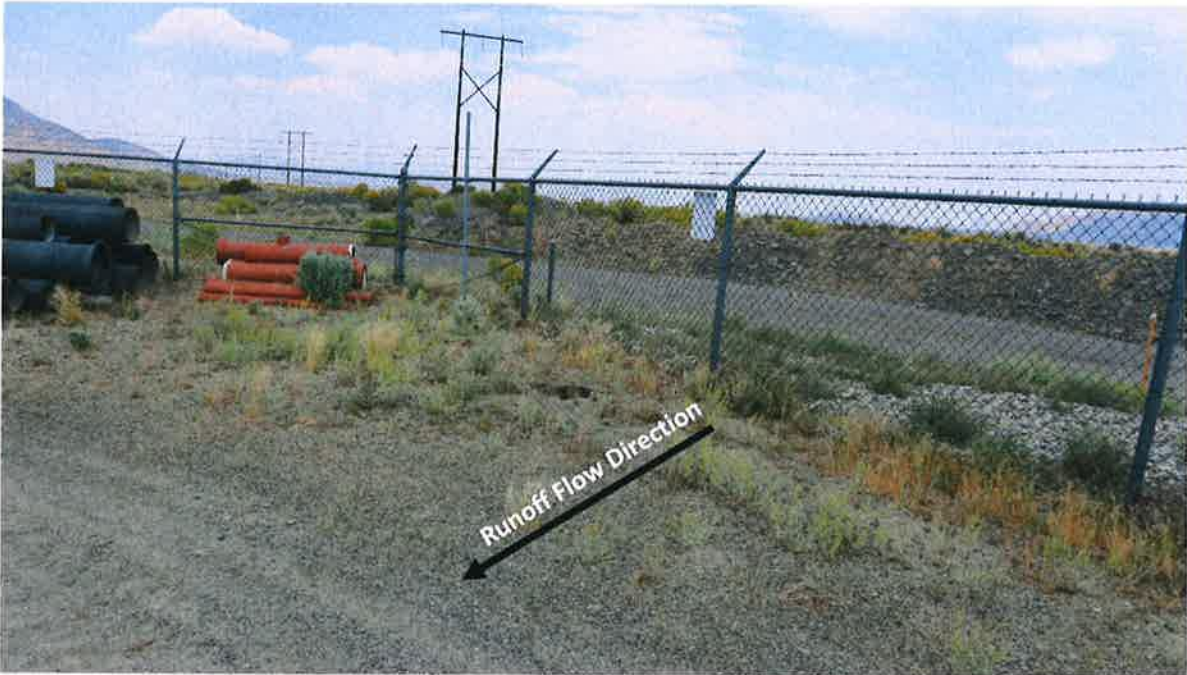
Figure 9: Inside of North Fence showing approximate 5-inch berm.
