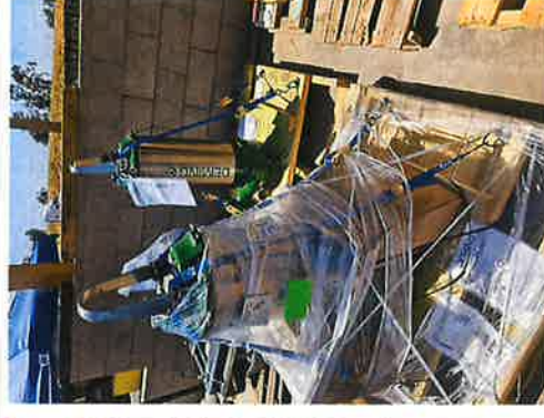
New pumps delivered
